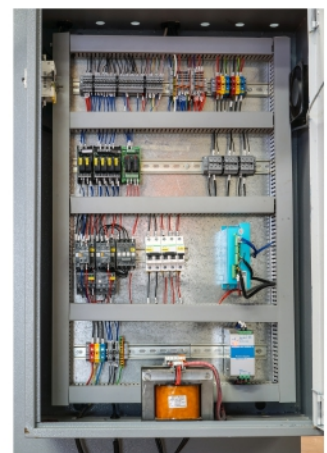
Electric Panel Schneider
